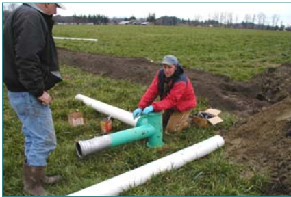
Cost share funds enabled over 100,000 feet of high pressure underground pipeline to be installed during 2001-2003. Here Darryl and Steve VanderHaak assemble a T-fitting with riser for manure application.
