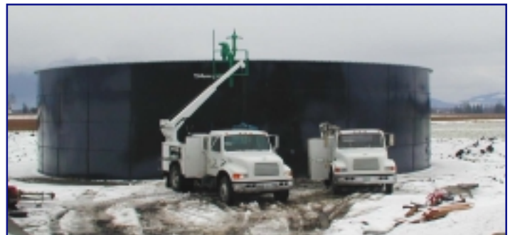
The District engineer facilitated design and installation of this manure storage tank, a BMP paid for through state cost share funds.
