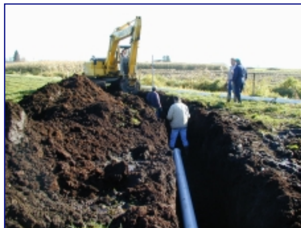
Crew installing waste transfer pipeline at dairy farm north of Lynden in Whatcom County.
